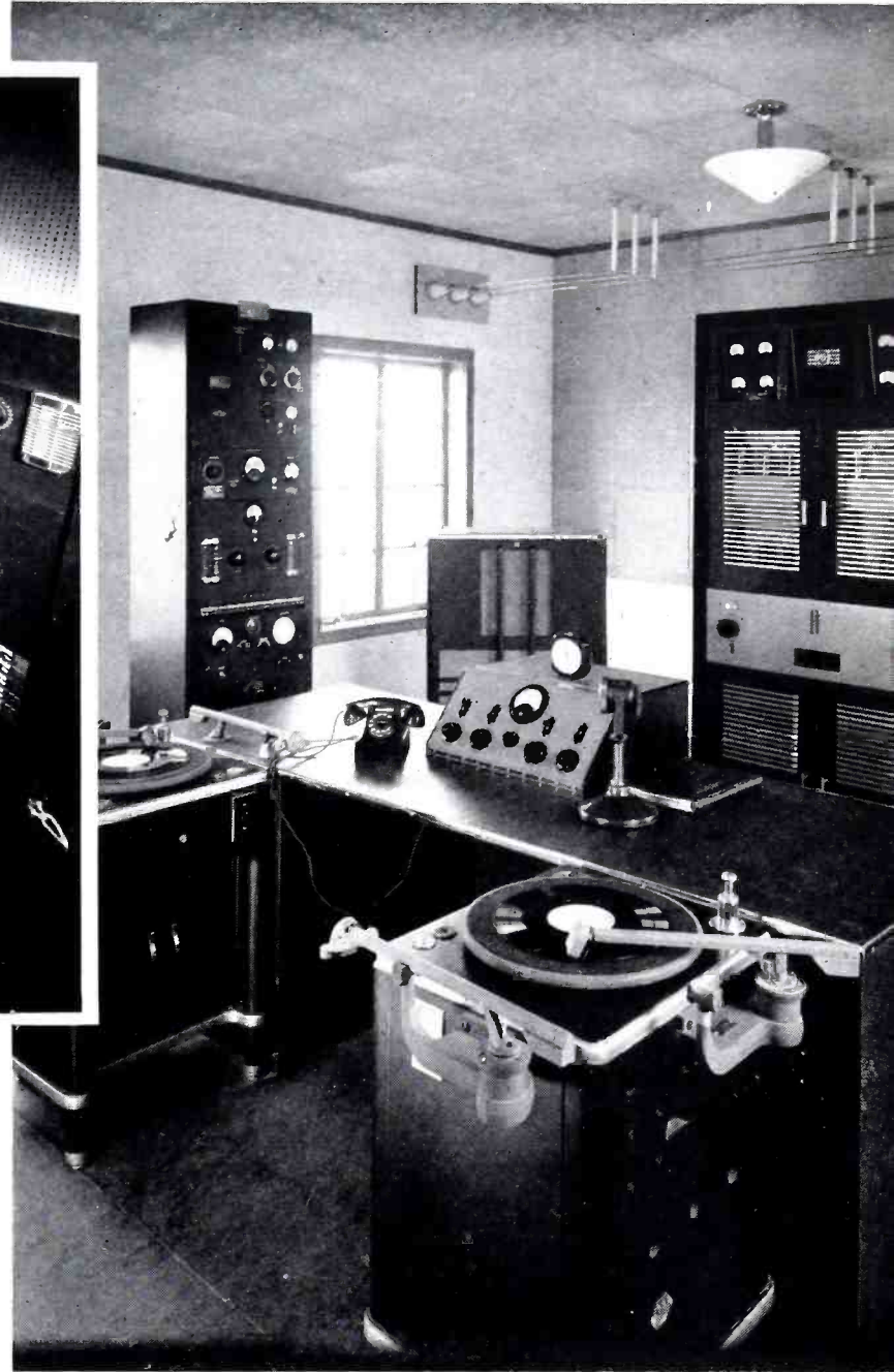
KARM Transmitter Plant.
